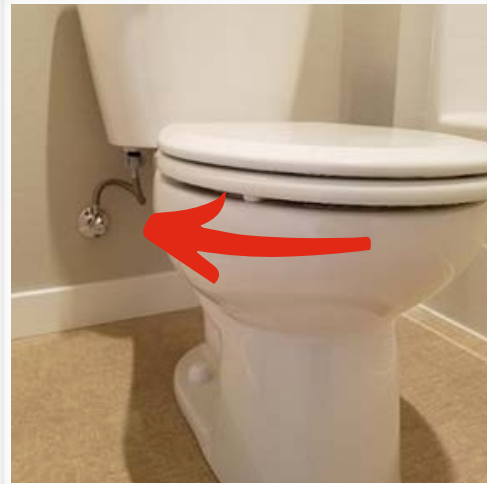
TOILET SHUT OFF
