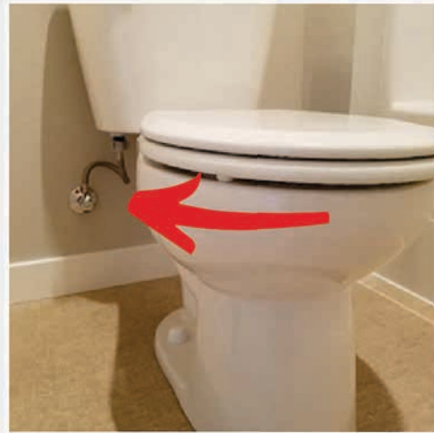
TOILET SHUT OFF
