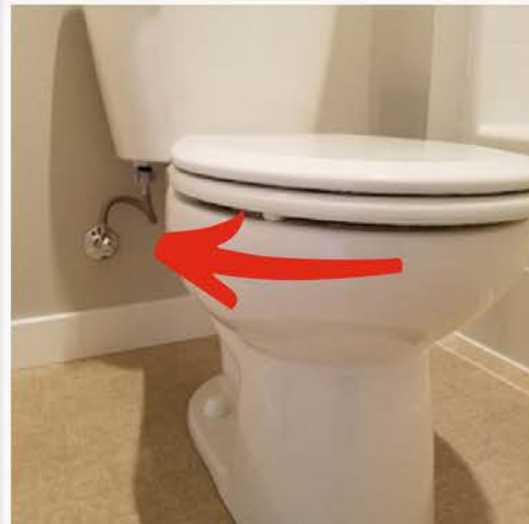
TOILET SHUT OFF
