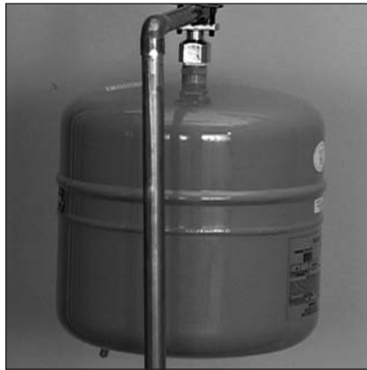
Figure 18 - The Thermal Expansion Tank should be pressurized with air to match the home's incoming water pressure.
