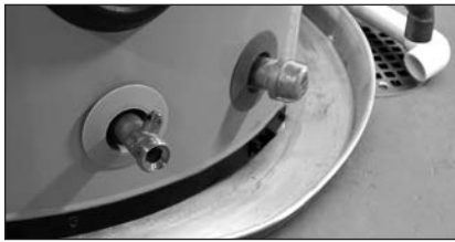
Figure 7 - A suitable drain pan piped to an adequate drain can help protect flooring from leaks and drips.
