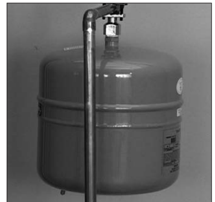
Figure 6 - A Thermal Expansion Tank helps protect the home's plumbing system from pressure spikes.
